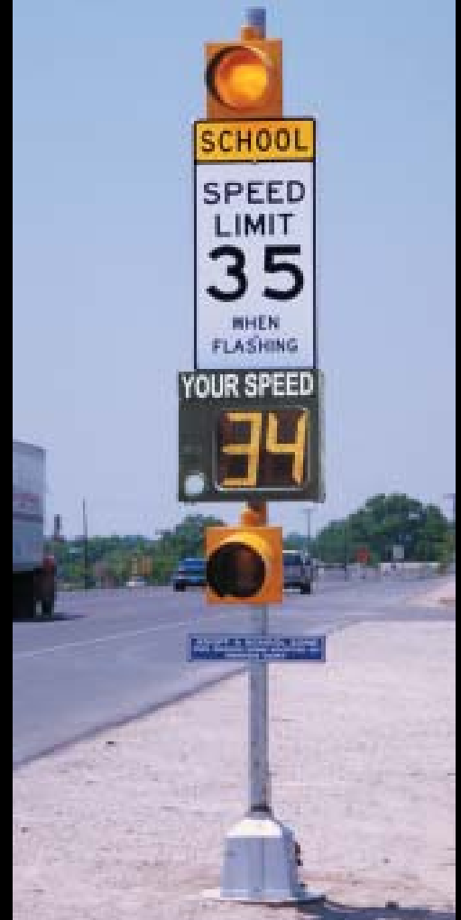
Mounted to existing AC-powered school zone pole.
